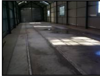
Left: Casting of the new floor complete. Since this photo was taken the floor has been sealed with paint and the shed is ready for its new inhabitants.
