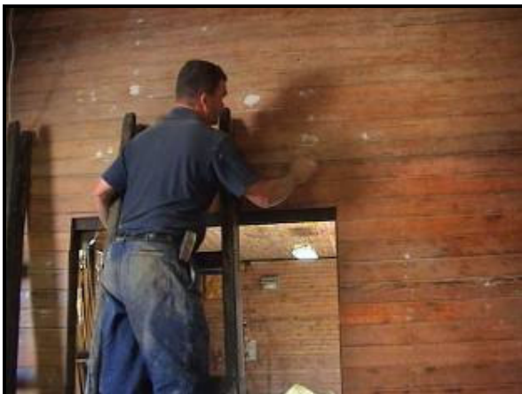
Above: Phil Pedley carrying out patching of the original lining boards in the centre room.
