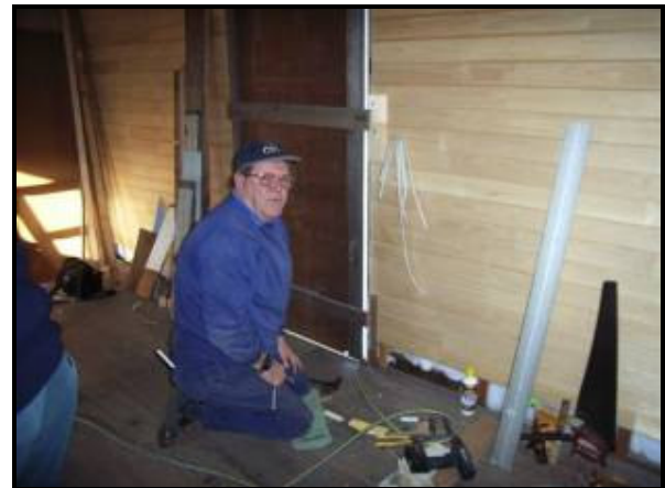
Above: John Parker placing packing pieces at the junction of the floor and the walls to support the skirting boards.
