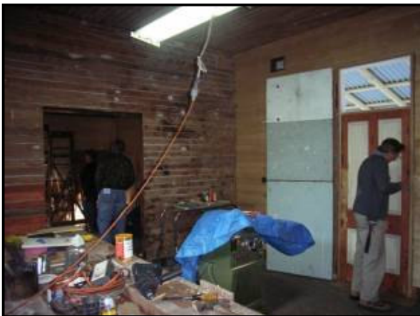
Above: Carpenter David Grove fitting the lock to the door in the centre room. Note the new boards on the right hand wall
