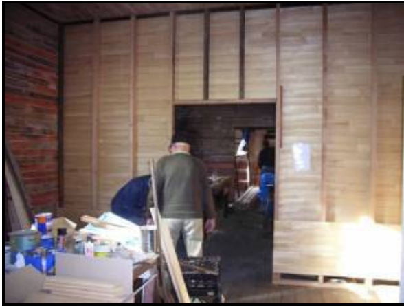
Above: In this image lining boards being fitted to the new partition wall between rooms 1 and 2. This wall was necessary to keep the interior architecturally correct in accordance with heritage requirements.
