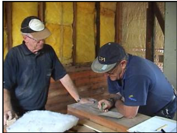
Above: Dennis Brown and John Parker sorting out a plan of attack for the next phase of the work.
