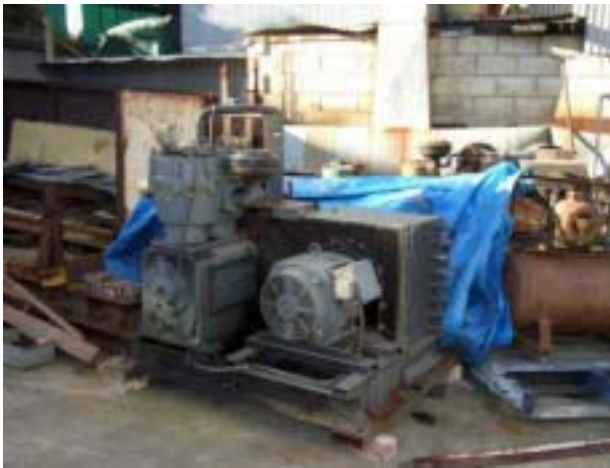
Pulford Air Compressor
