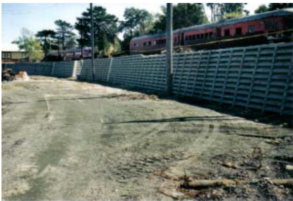
Retaining Wall completed in preparation for STaRPS new Shed. Photo: Andrew Teste
