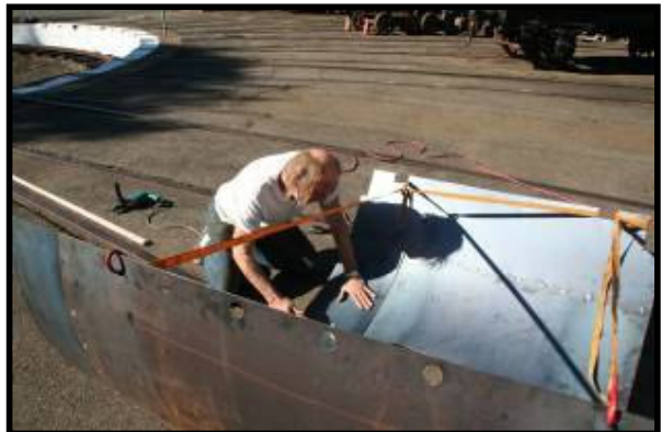
Above: Stephen Dive shapes the final sheet of Boiler Cladding for 5461 prior to it being painted and fitted to the Locomotive. (Photo: Rod Hawkes).
